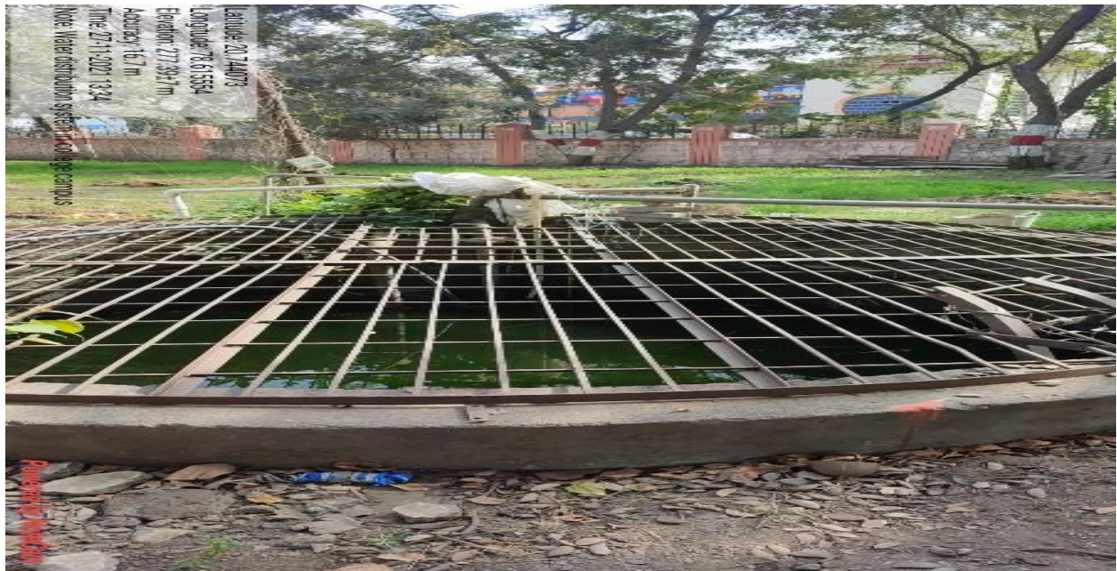
Figure: Water distribution system (well water distribution) in college campus
