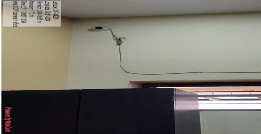
Figure – CCTV camera in office
