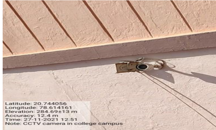
Figure – CCTV camera in college campus
