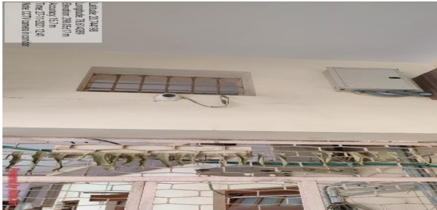
Figure – CCTV camera in corridor
