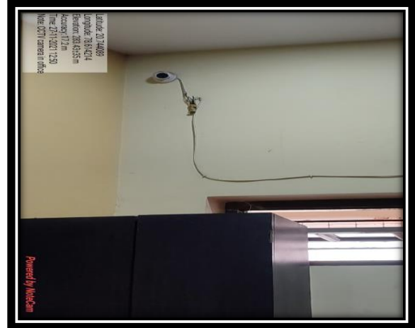
CCTV camera in office
