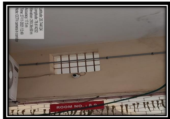
CCTV camera in corridor
