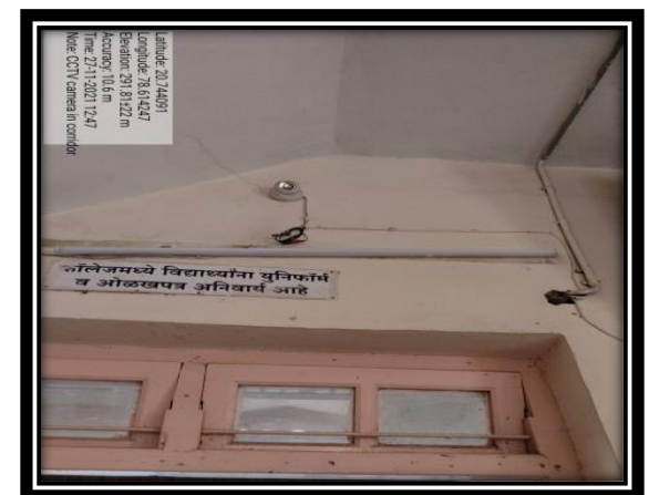
CCTV camera in corridor
