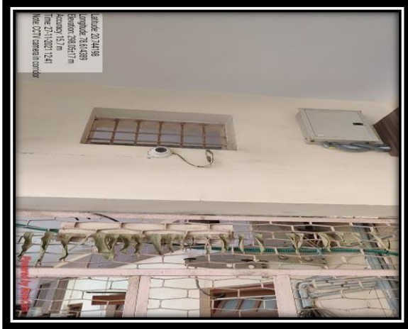
CCTV camera in corridor
